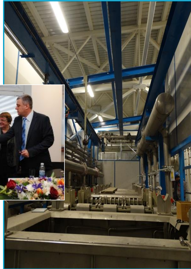
Size Reduction and Decontamination Facility
